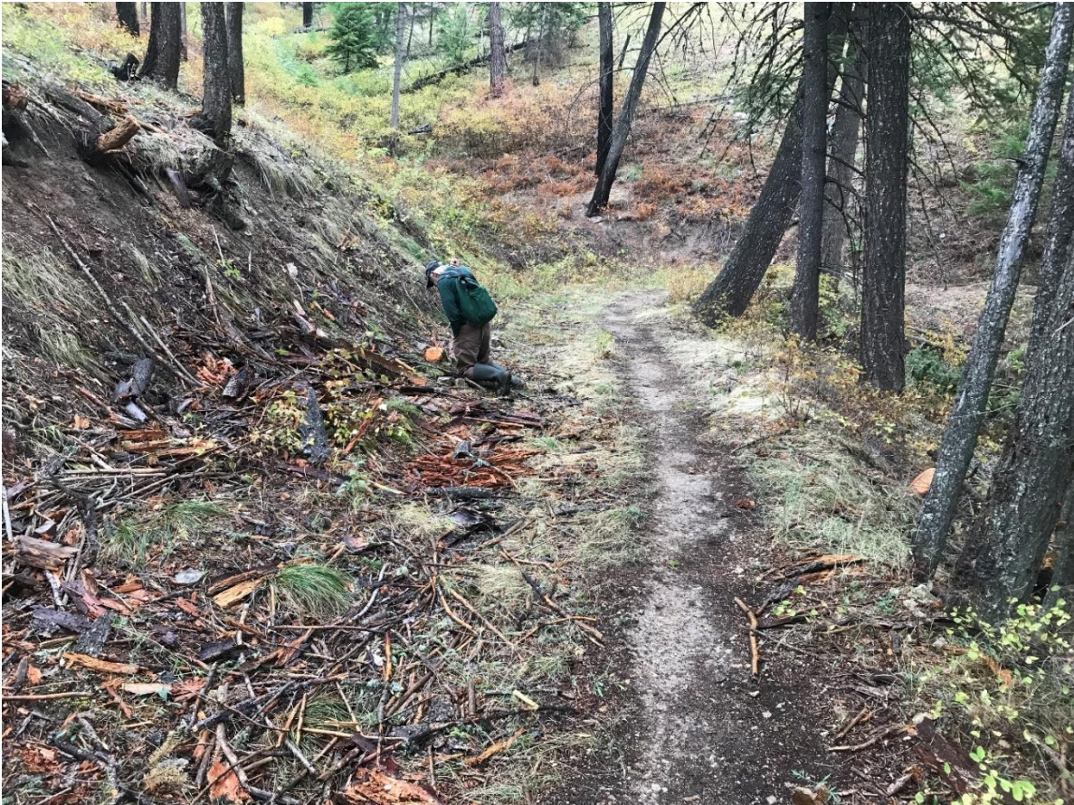
Hand line cut along the old irrigation ditch several hundred feet west of the commercial logging area, rehabbing the 2000 fire line. Dead trees and downed logs were cut up, and live trees were limbed. This work here was done after the commercial logging farther east had begun, according to local residents. In the Bodgett Creek area, where there
